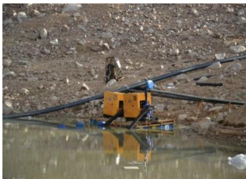
Pump mounted on a floating platform (A. P. Medeu et al., 2020)
