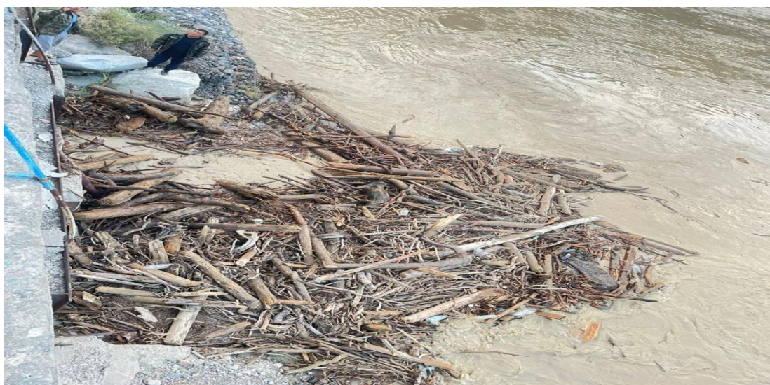
Figure 3. Consequence of mudflow on 21 July 2023 at the dam of Talgar river (photo 22.07.2023 by 'Kazselezaschita').
